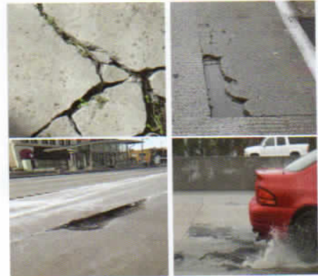
Water-related damages: potholes, corner breaking and wide cracks
