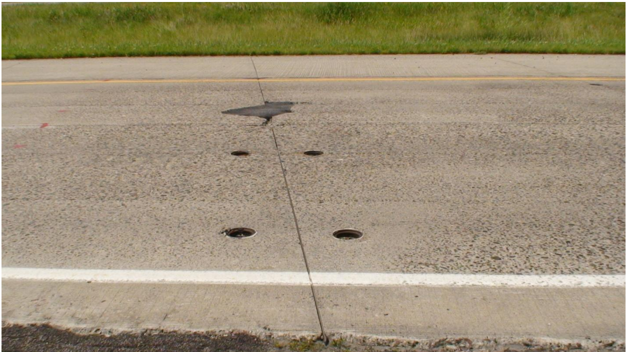
Figure 6 Open Instrumentation Hand Holes on MnROADS Sections
