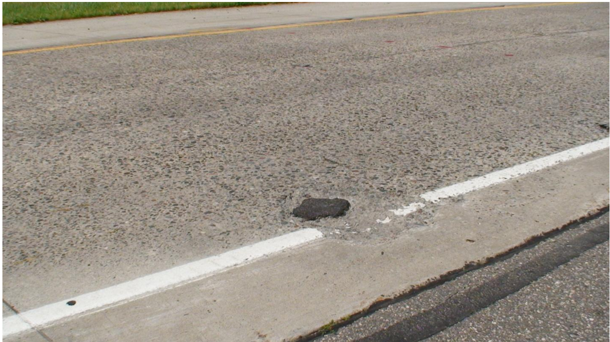
Figure 4 Pothole in Cell 8 CDG Causing All Testing to Be Shifted to Left Side of Lane
