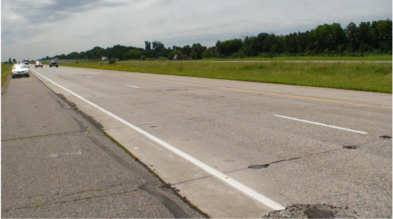
Figure 5 Distress Evident on I-94 Cell 8 CDG
