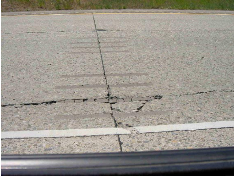
FIGURE 6 Longitudinal cracking in dowel bar slots.
