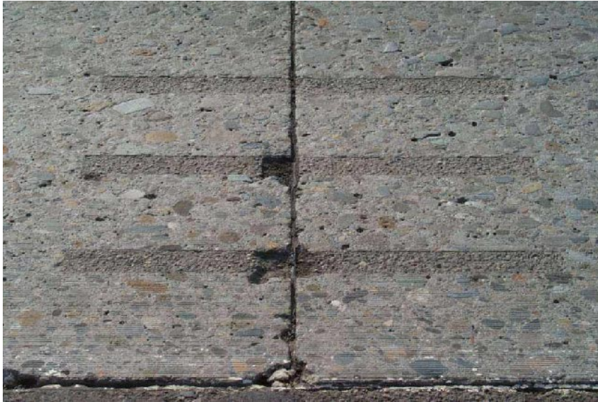
FIGURE 8 Joint spalling due to misaligned core board.
