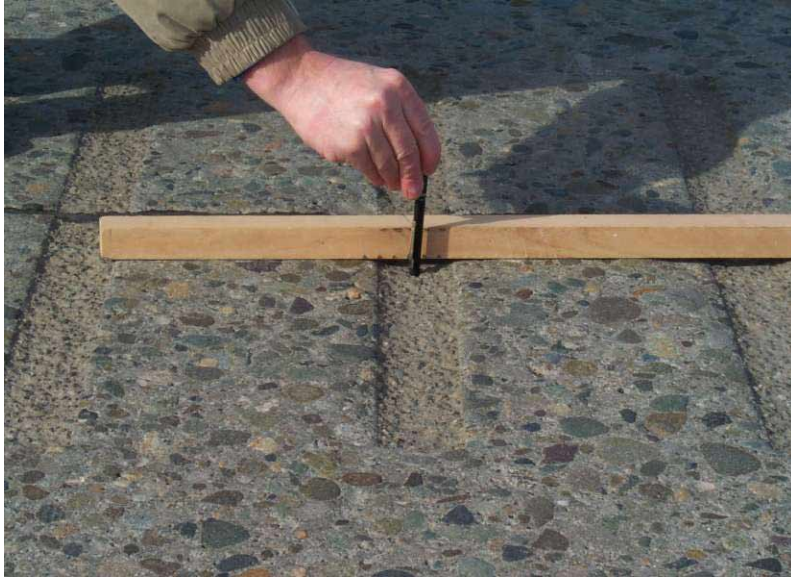
FIGURE 5 Example of accelerated wearing of grout in dowel bar slot.
