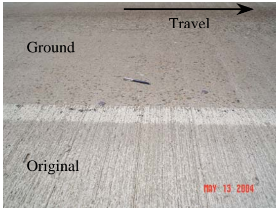
Fig. 10: Photograph of the northbound bridge deck on I-5 showing the ground travel lane and original texture shoulder
